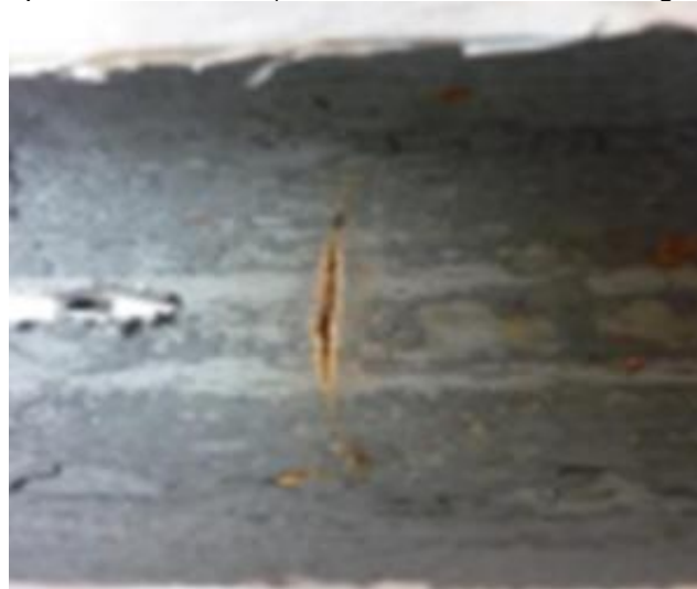
Figure 9: Material that has cracked resulting in a hole
