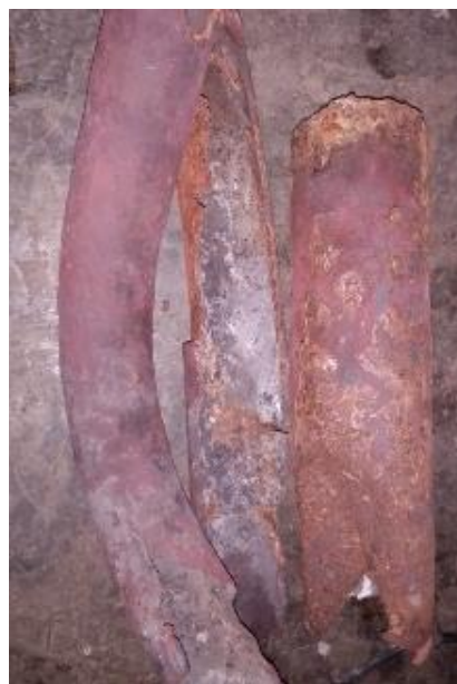
Figure 6. Pieces of pipe that have failed/damaged
