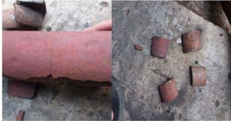
Figure 4. Pipe pieces that have undergone combustion activity
